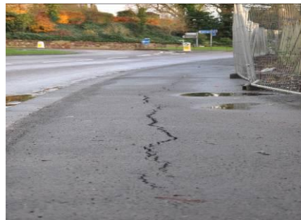
Cracks in the pavement
